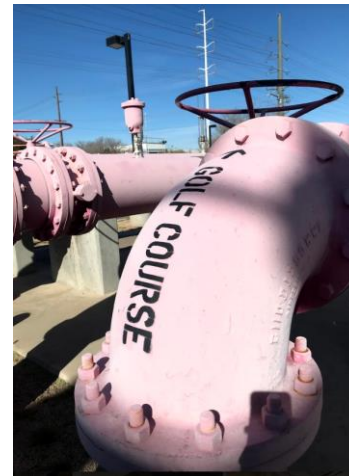
Figure 8: 1 of 3 Distribution Pipelines (Team Photo)
